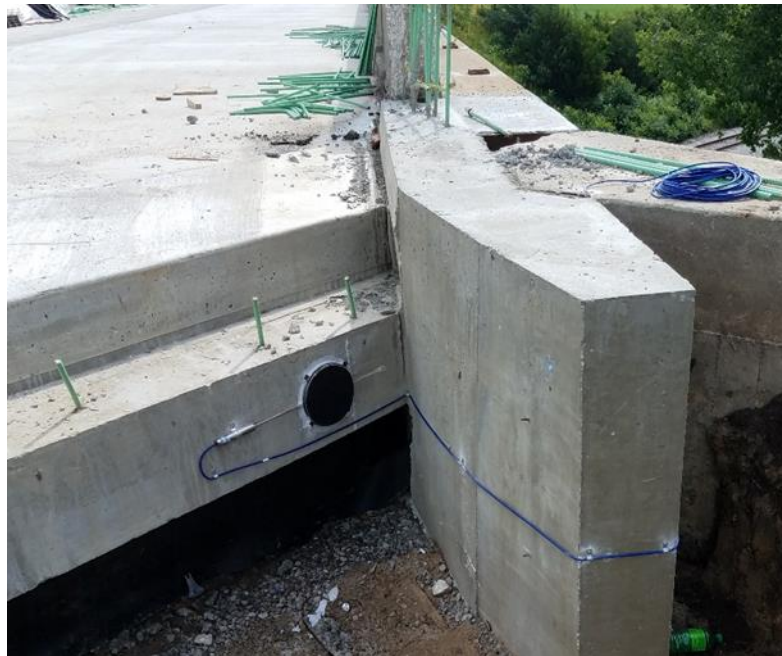
Figure 5.4. Jasper - EP1-W Earth Pressure Sensor after Installation
