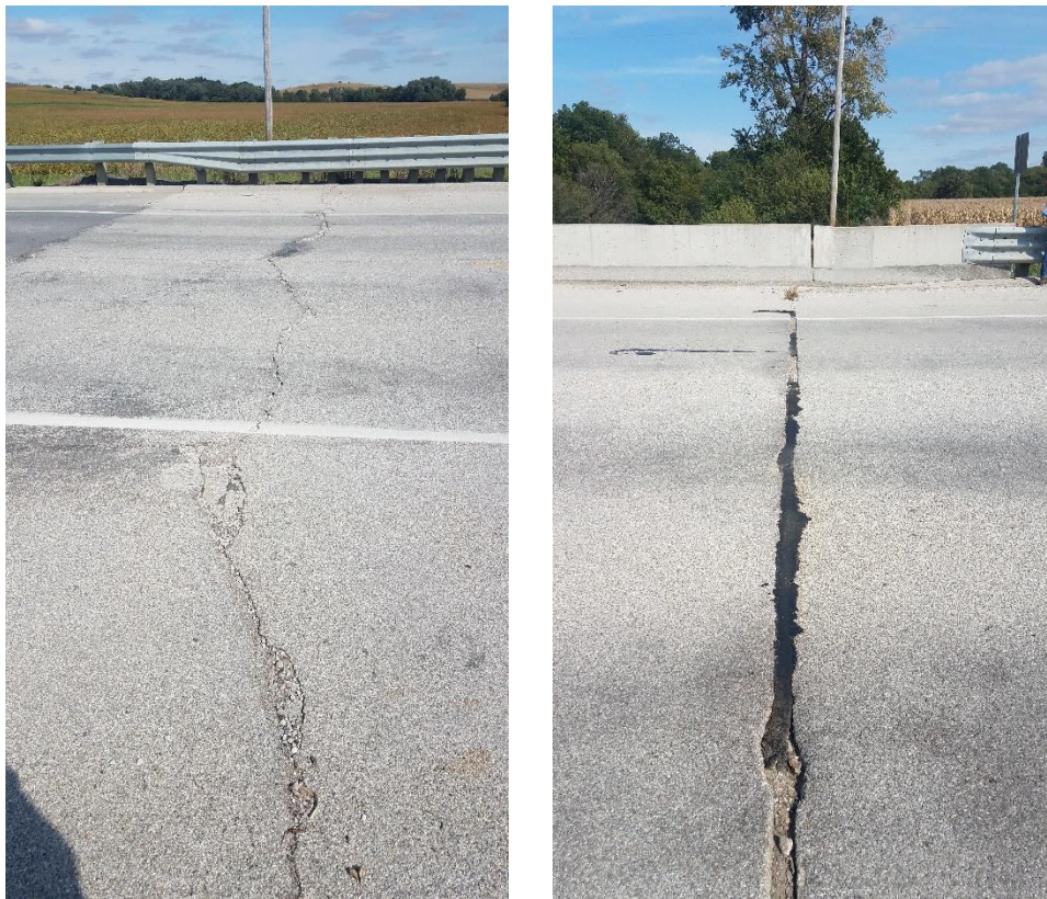
Figure 4.3. (a) Transverse Approach Slab Crack (left), (b) Bridge Deck to Approach Slab Joint (right)
