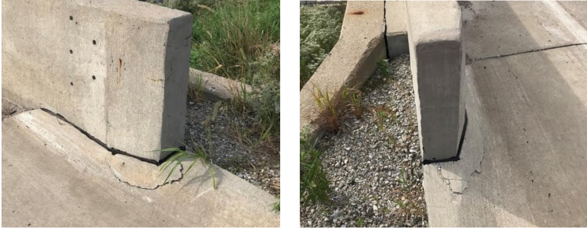
Figure 4.8. (a) Concrete Cracking at the end of the Wingwall (left), (b) Additional Cracking at the end of the Wingwall (right)
