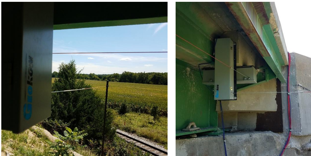
Figure 5.7. Jasper - (a) Displacement Transducer with Reference Post (left), (b) Longitudinal and Transverse Displacement Transducers Attached at the Acute Bridge Corner (right)
