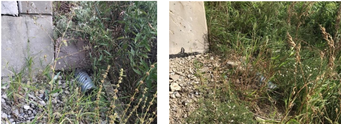
Figure 4.9. (a) Blocked Embankment Drainage (left), (b) Additional Blocked Embankment Drainage (right)
