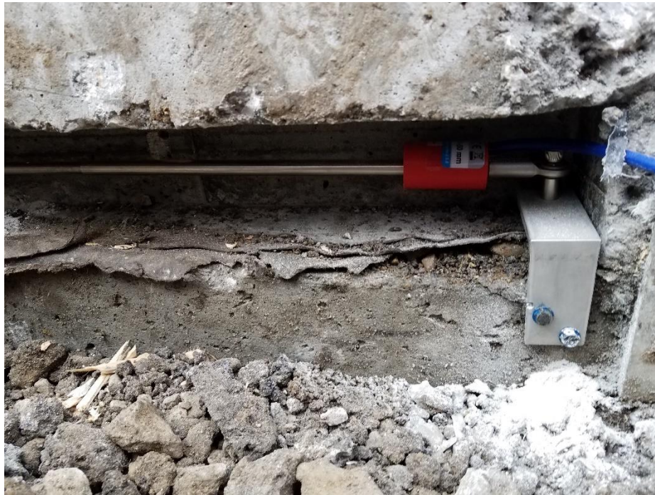
Figure 5.28. Story - Crackmeter Approach Slab Side Blockout Location
