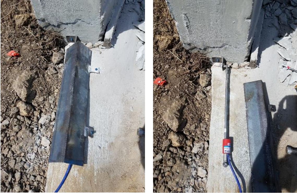
Figure 5.6. Jasper - (a) Crackmeter without Protective Cover (left), (b) Crackmeter with Protective Cover Installed (right)
