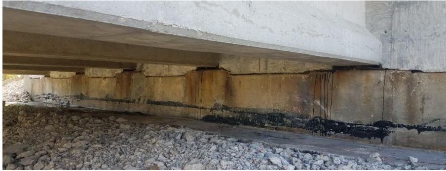
Figure 4.7. Abutment Face Showing the New Backwall on top of the Old Footing
