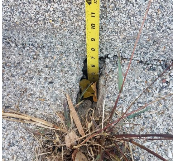
Figure 4.4. Void at the Intersection of Deck to Approach Joint and Barrier
